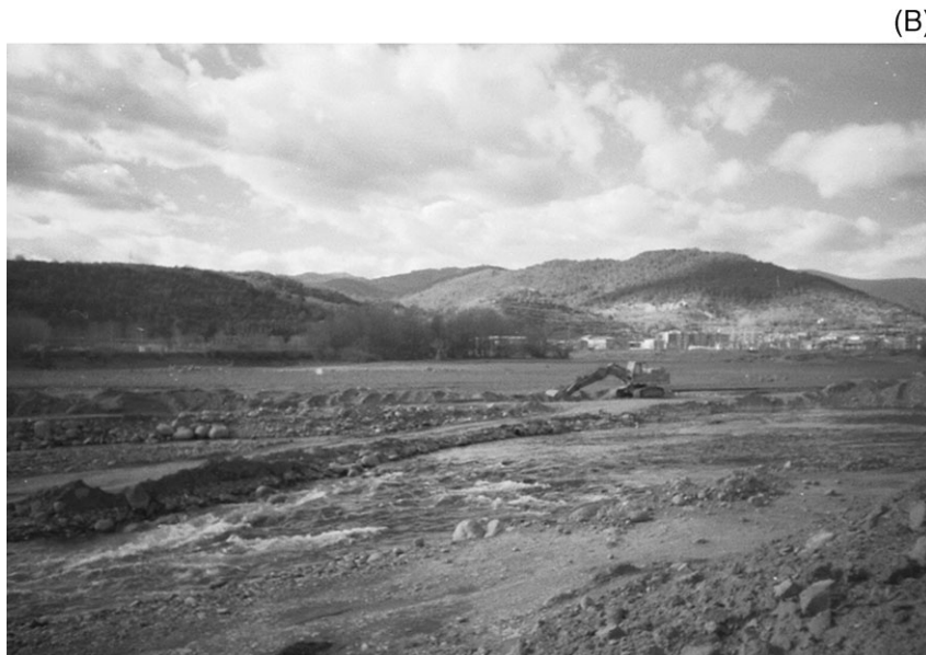
Figure 4. (A) Sedimentation (content: silt 76%, clay 19%, coarse fractions 5%) in the Barasona reservoir (Ésera River, Ebro basin, Spain), which has been in operation since 1932. (B) Mechanical extraction of sediments in the delta of the Talamà Reservoir (Noguera Pallaresa River, Ebro basin, Spain). This has been practised since 1990 (photo (A) by R. J. Batalla (June 2001) and photo (B) by J. Caba (June 2002). The photo in (A) is reproduced with kind permission of the Spanish Society of Geomorphology and the Spanish Quaternary Association)
