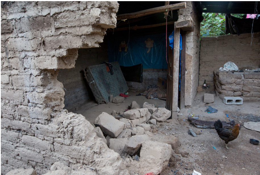
An abandoned home in La Cuchilla, that crumbled and partially caved in due to tremors caused by the use of explosives in Tahoe's tunnels. San Rafael Las Flores municipality, Guatemala.
